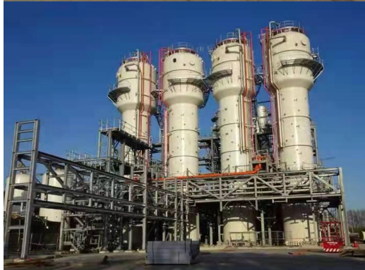
Bio-Reactors Steelanol Project- Geel Reactors 4 Sets DN5800/7400*70000 SA516 Gr.70N / SS
