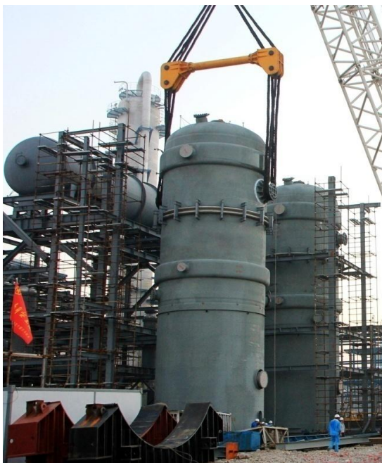
Synthesis Gas to Glycol Unit Coupling Reactor DN6000, 497tons 17,793 tubes, SS304
